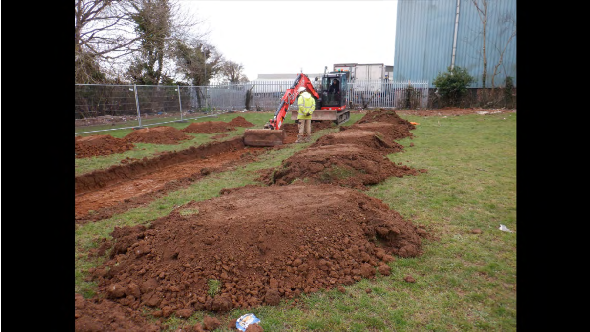
Plate 15, E facing working shot of excavation of Trench 9.5, showing UKPN works fenced off to the NE of the trench.
